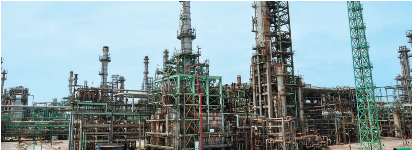
ISOM Plant of Euro IV Project at a Refinery in Manali
