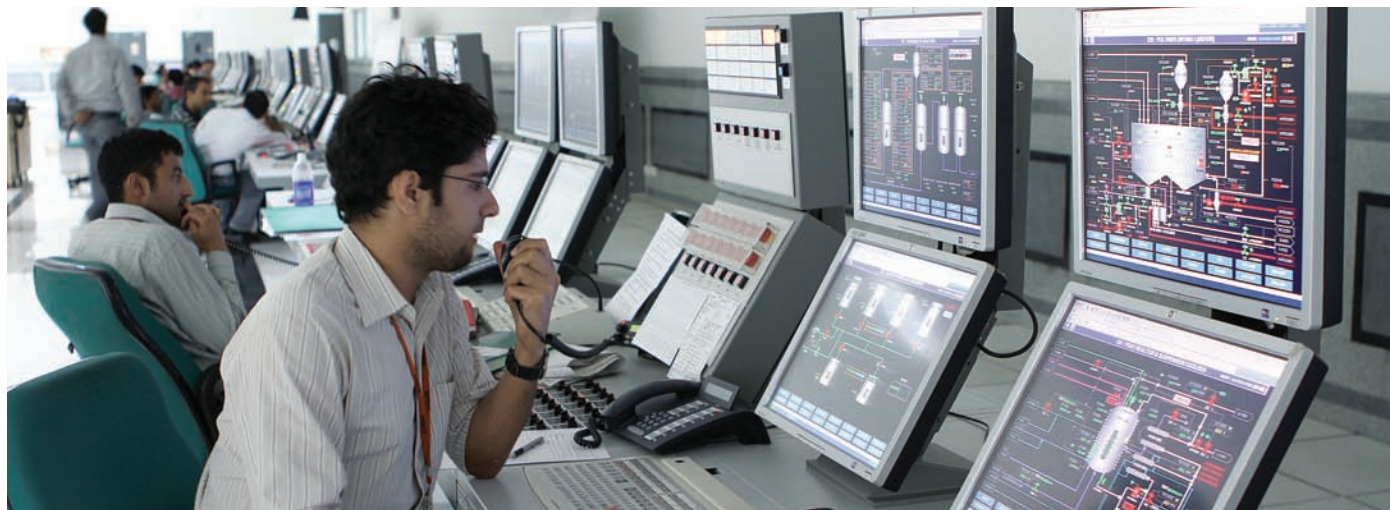
State-of-the-art control & monitoring room in a Refinery
