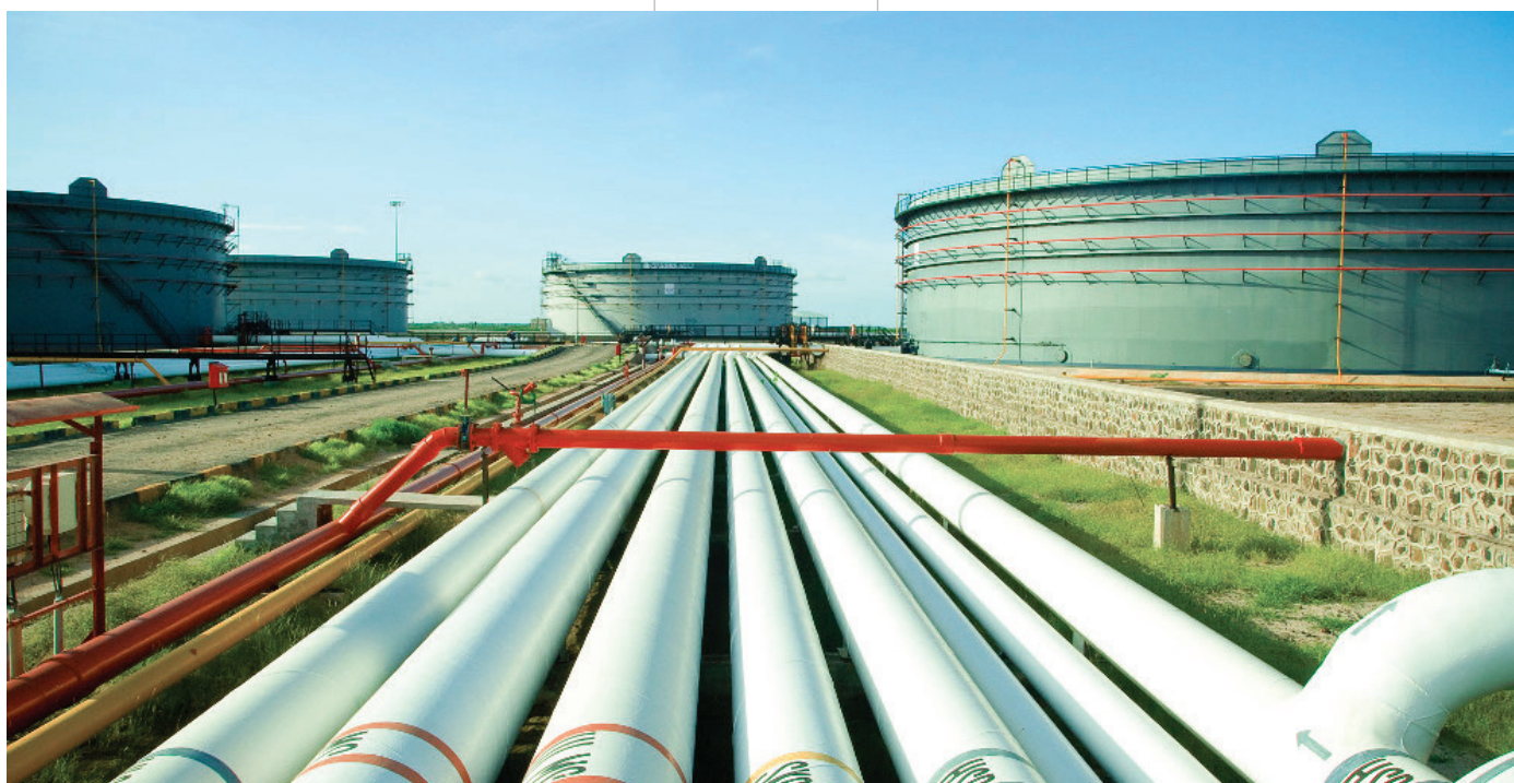
Pipe racks at a terminal in Jaipur
