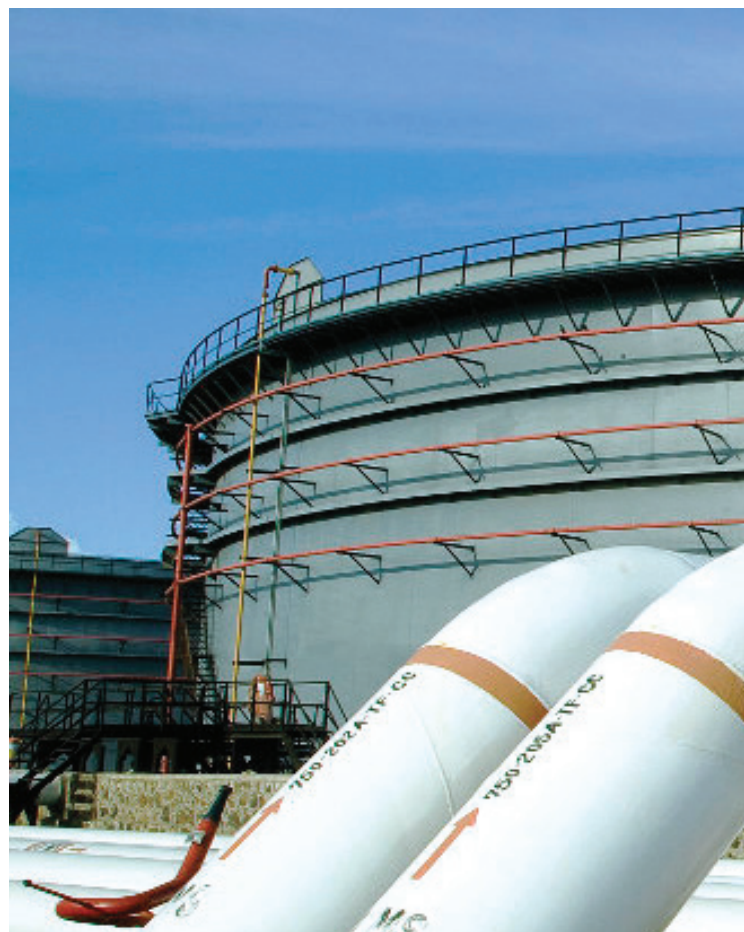
Pipe rack for different grade of products
