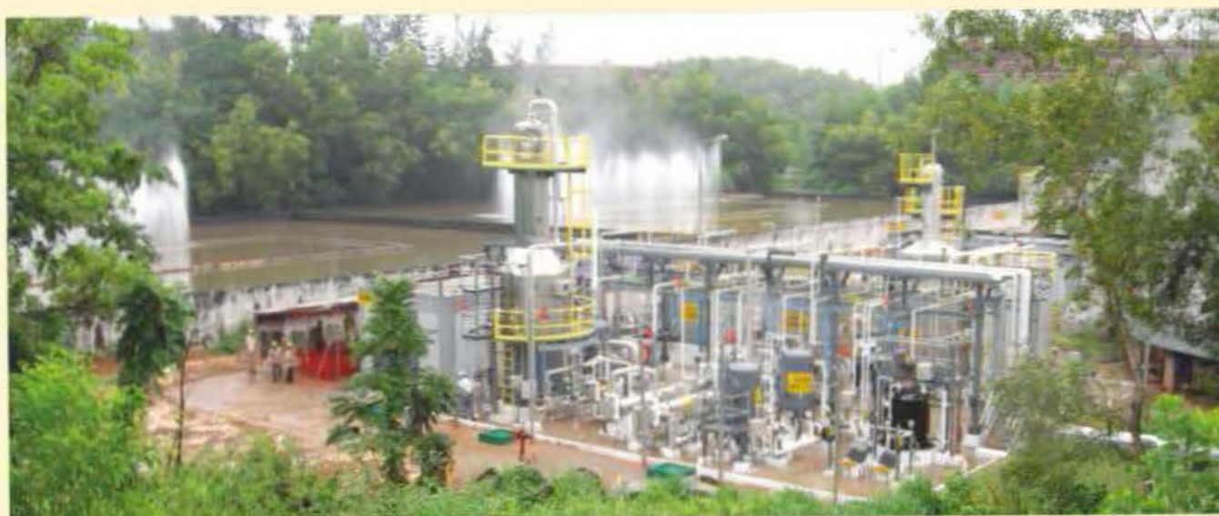
Wet Air Oxidation Plant, MRPL
