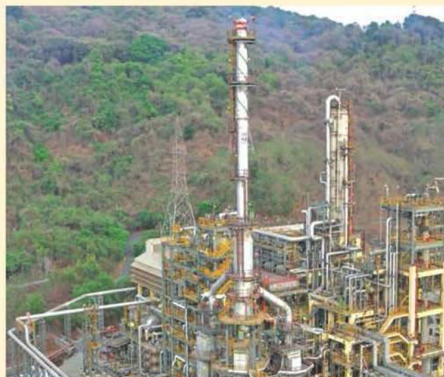
HPCL's LOBS quality upgradation plant
