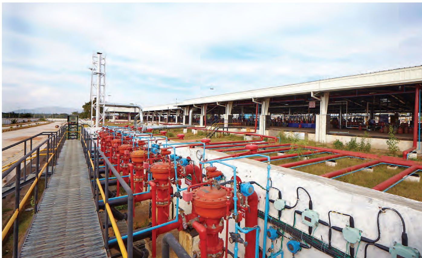
IOC LPG Refinery, Mysore
